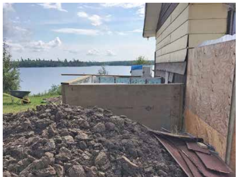
Phase 4 of the water retrofitting continued throughout the whole week we were there.
