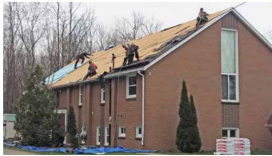
Above: Spring roofing: The roofers started their work on April 18, 2019, Maundy Thursday. The congregation held their worship in the basement.
