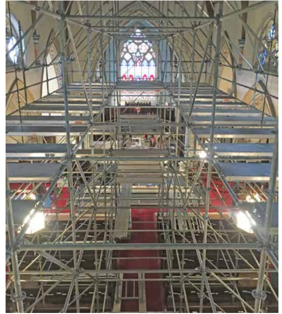
A giant scaffold was installed and disassembled in the church between Sundays so that the upgraded lighting and fans could be installed 50 feet up from the floor.
