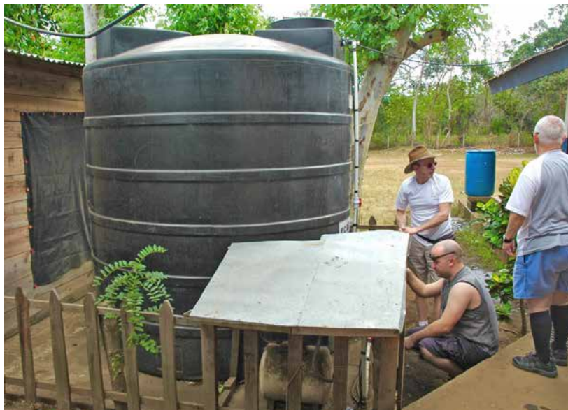
▲ Rob Simmons, Tom Pollard, Roy Simmons installed a 10,000 litre water tank and purification system to provide safe drinking water.
