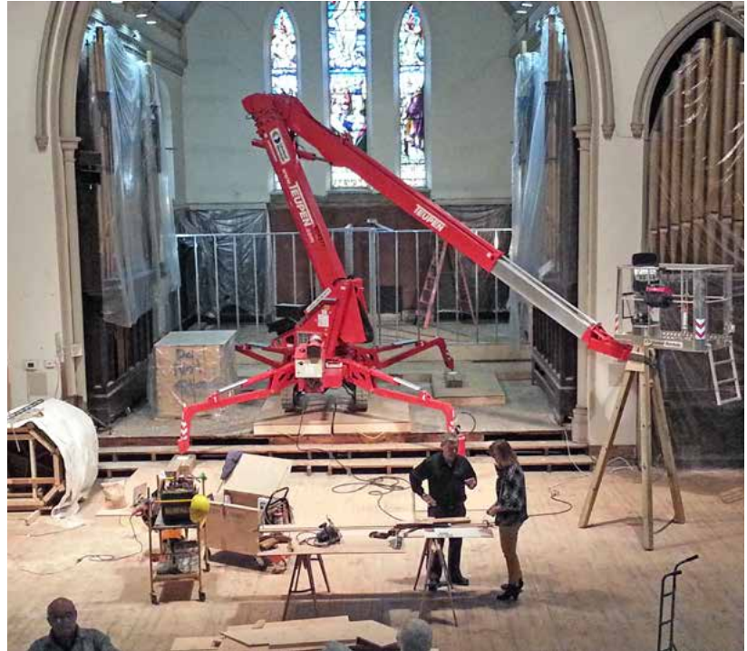
The "spider" safely lifted workers high enough to repair and paint all the walls of the Church of the Ascension Hamilton.
